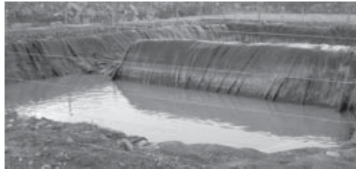
Holding pit for well drilling discharge prior to disposal off site.
