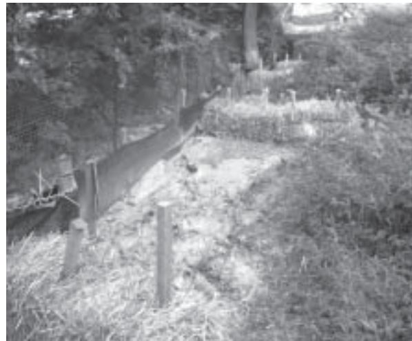
Silt fence installed down a hill, hay bales added to try to check flow, and failing rock filter at bottom of hill
