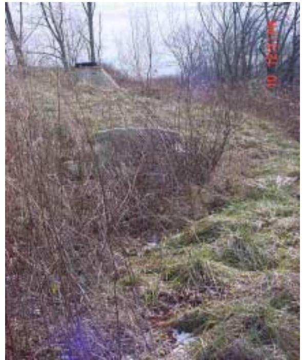
This trench has a subsurface energy dissipator to reduce the velocity of entering stormwater.
