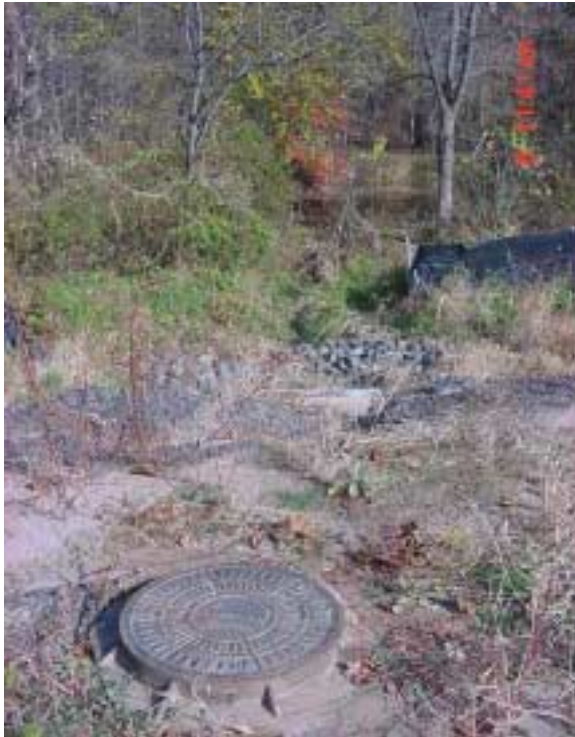
Manhole access to stormceptor® chamber below ground.
