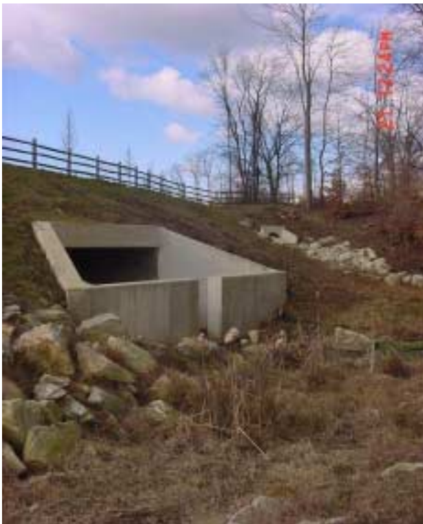
The vegetative swale converges with Shamona Creek and flows under the road.
